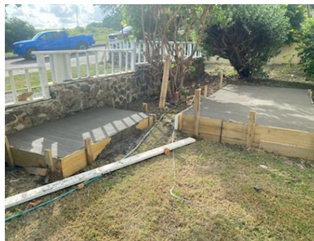
Concrete pad for generator & fuel tank
